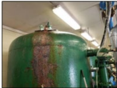
Figure 13 - Tank Manway Rust
