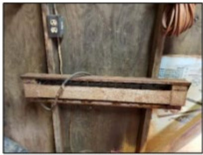
Figure 1 - Well House Heater
