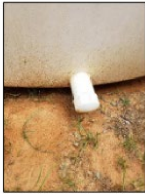
Figure 2 - Backwash Tank Drain
