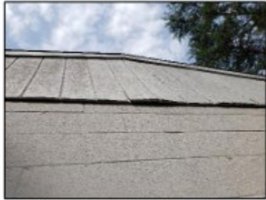
Figure 7 - Roof Trim Peeling
