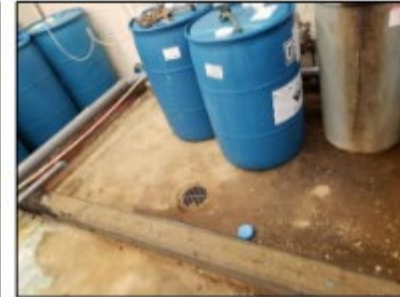
Figure 11 - Chem System Containment
