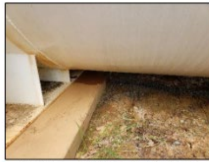
Figure 3 - Backwash Tank Support
