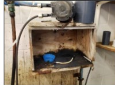
Figure 10 - Chem Pump Shelf
