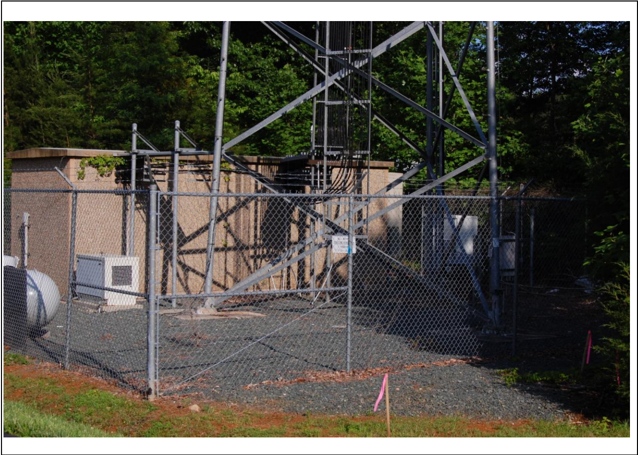
Figure 3: Example of 800 MHz Base Station
