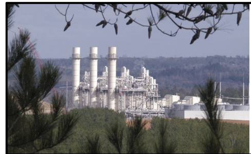
Figure NE-8, Tenaska
